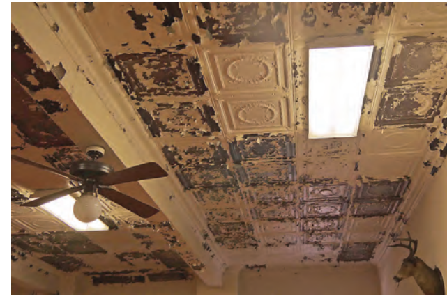
The ceiling in the Lodge Room has had repairs for numerous leaks but the historic tin squares on the ceiling are awaiting the appropriate and difficult historical renovation.
