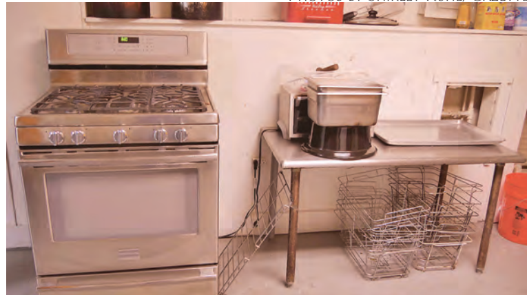
The most urgent need is a complete kitchen renovation from ceiling to floor including electricity and plumbing.
